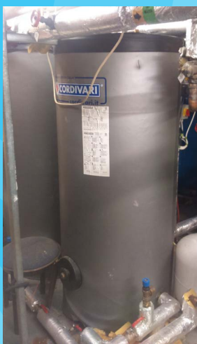
Hot water storage tanks
