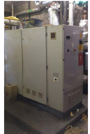
Old CHP unit
