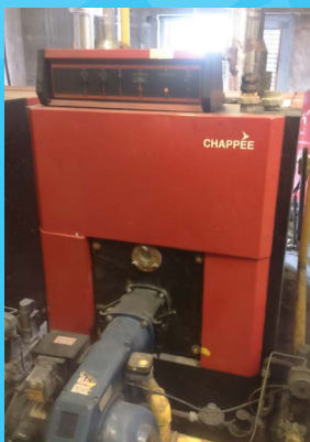
Natural gas boiler
